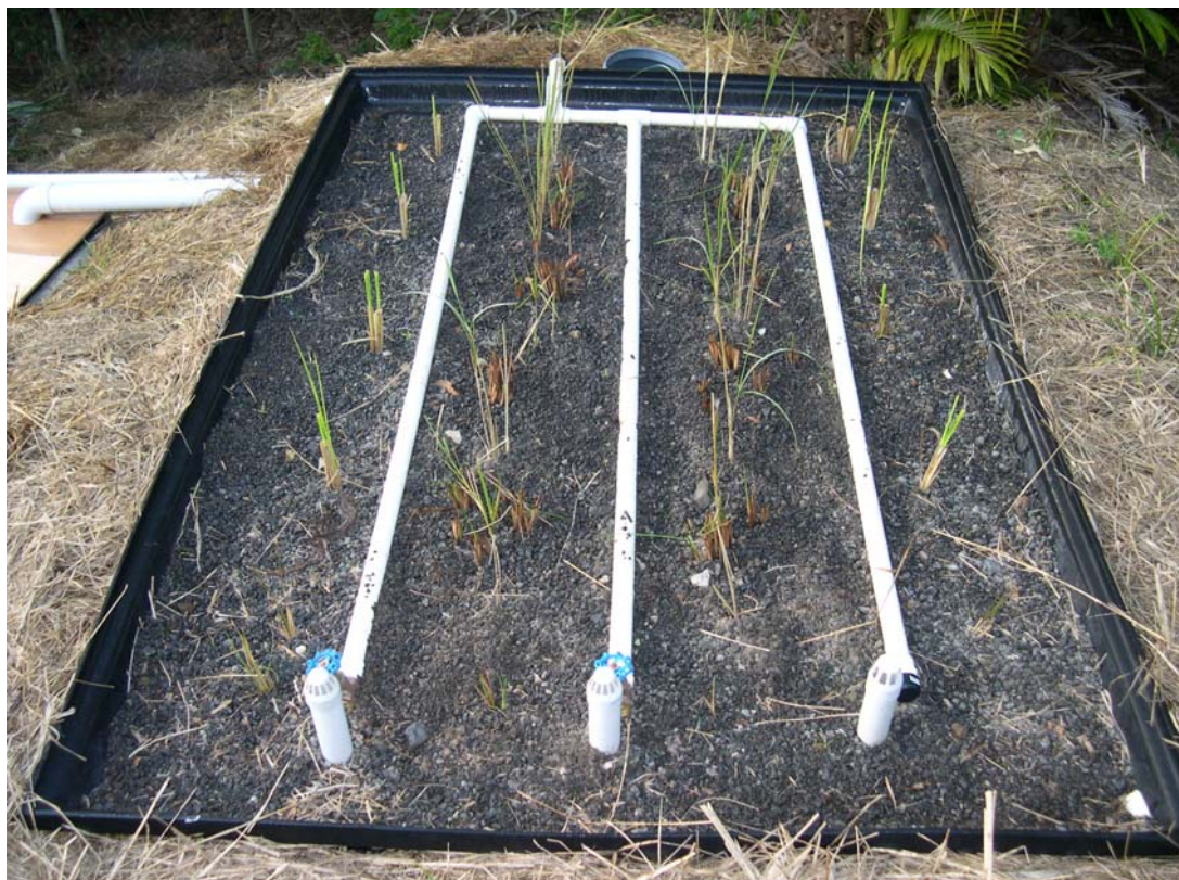
Figure 9. Wastewater distribution at vertical flow (VF) CWs at Bexhill, NSW, Australia. Photograph taken by the author.
